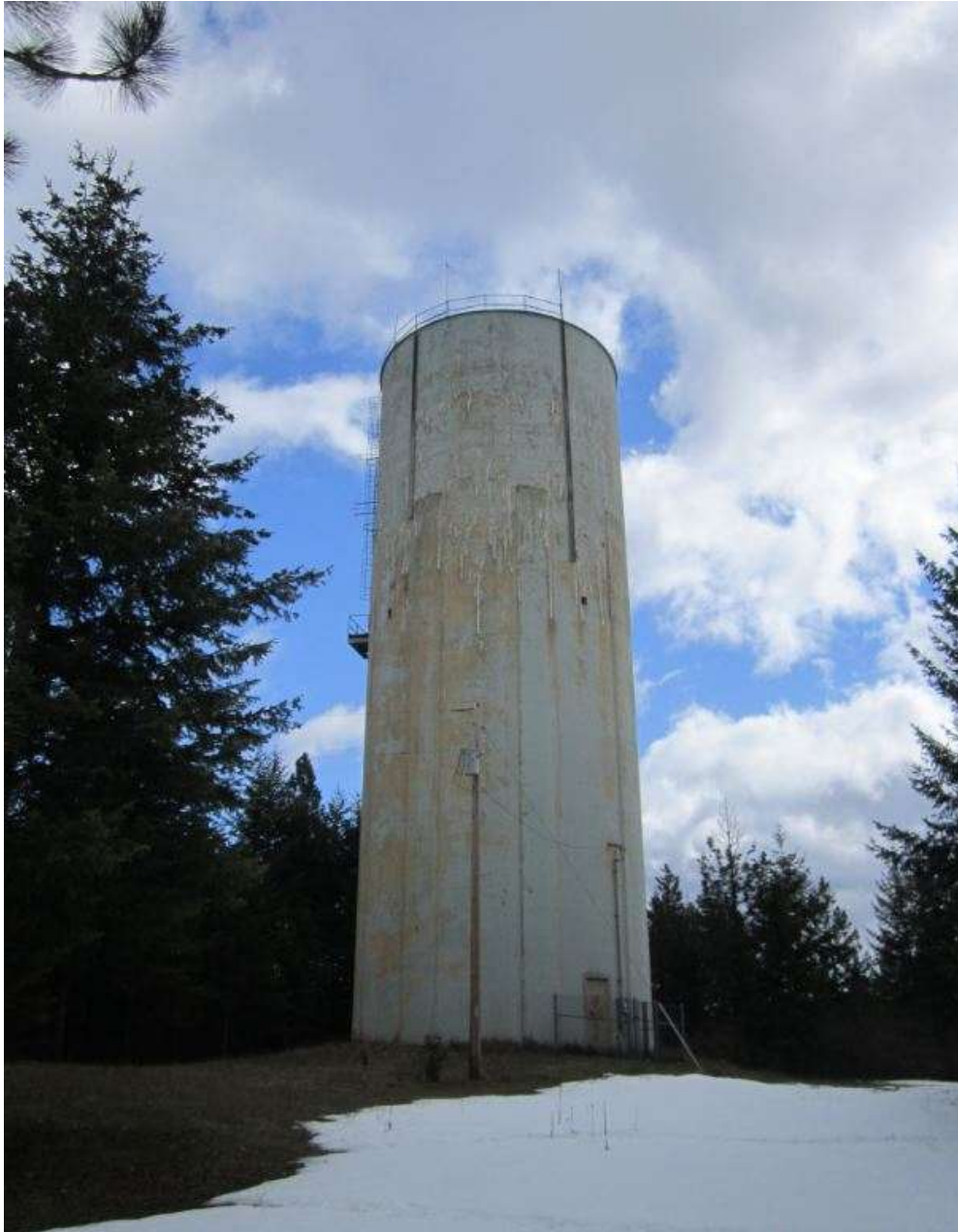
Figure 3. Farragut Reservoir Tank (225,000 gal)-July 2019
