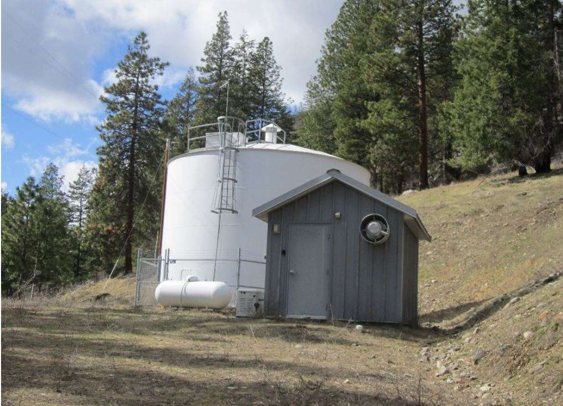
Figure 4. Pend Oreille Pines Tank (100,000 gal)
