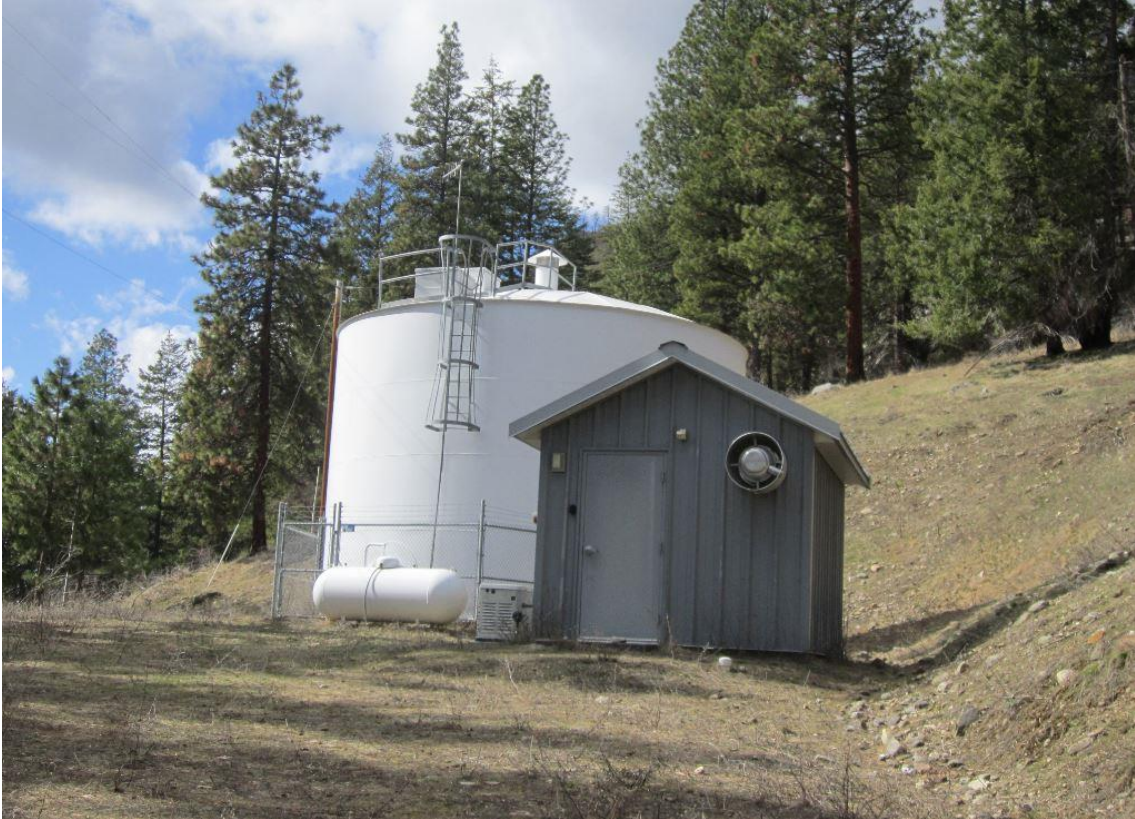
Figure 4. Pend Oreille Pines Tank (100,000 gal)
