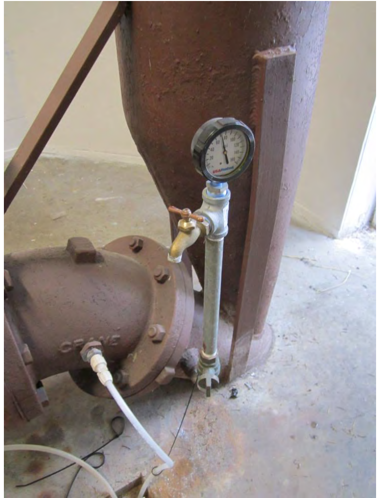
Photograph 20: Well 8 discharge appurtenances
