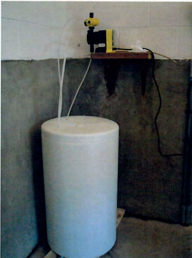
Photograph 11: Sodium Hypochlorite solution tank and LMI meter
