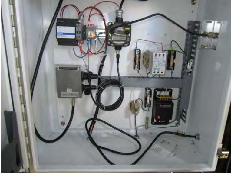
Photograph 33: Farragut Tank PLC SCADA relay/radio equipped w back-up battery
