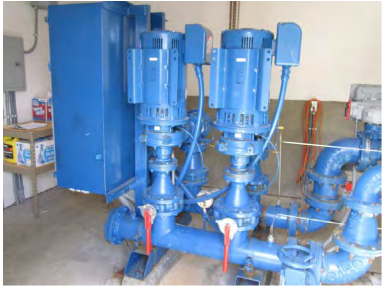
Photograph 66: Limekiln booster pumps
