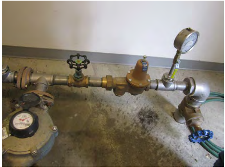
Photograph 62: Pend Oreille boosted discharge
