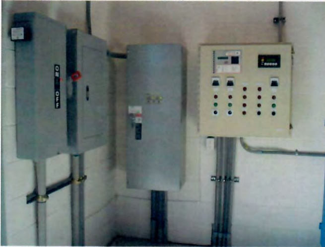
Photograph 9: Cape Horn Power Controls
