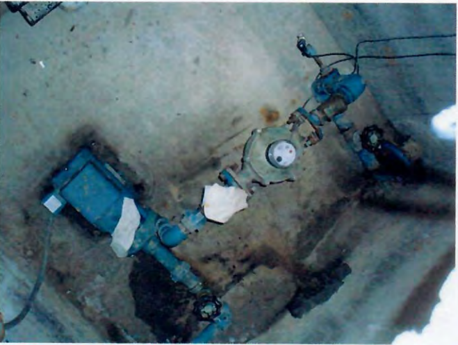
Photograph 17: Cape Horn Estates Booster vault
