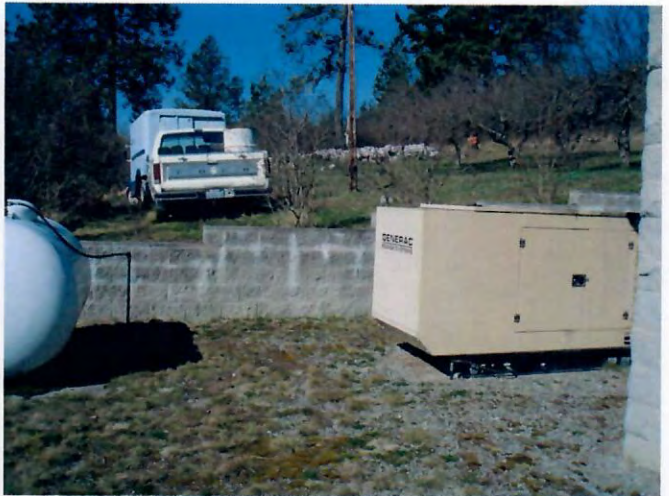
Photograph 8: Cape Horn Emergency Power Generator
