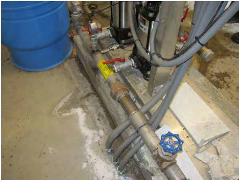
Photograph 63: Pend Oreille booster pump isolation valves
