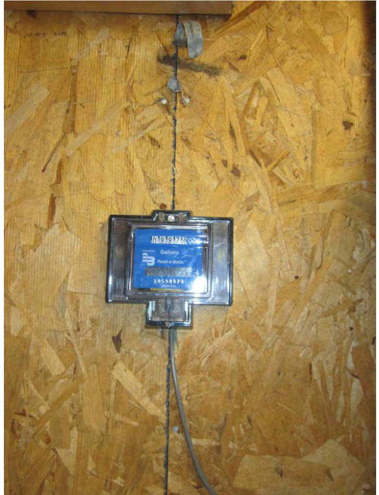
Photograph 40: Cape Horn booster station flow meter
