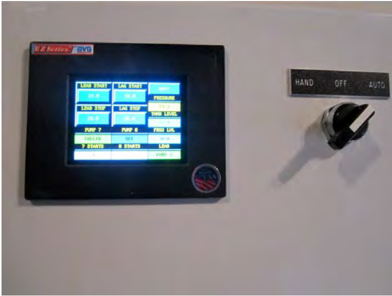
Photograph 11: Well 7 PLC tied to SCADA relay
