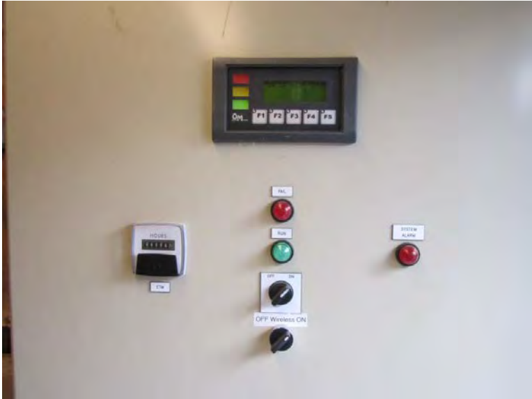
Photograph 39: Cape Horn booster station vault
