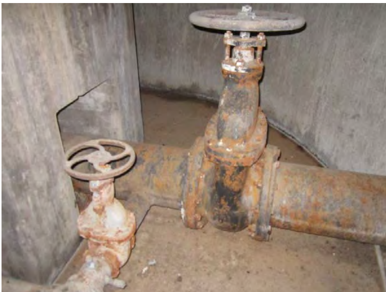
Photograph 29: Farragut Tank isolation valves
