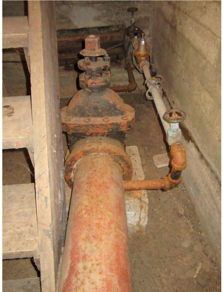
Photograph 48: Farragut tank PRV by-pass
