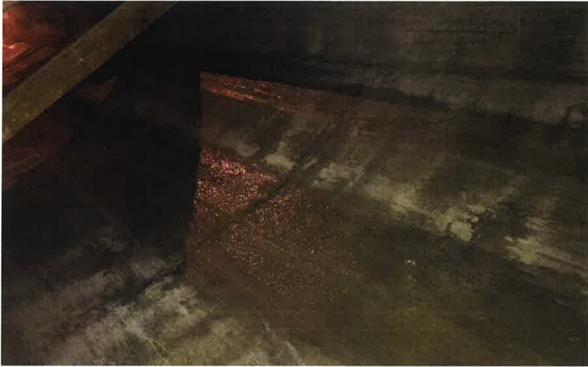
Figure 5 – Water Seeping Down the Interior Face of the Reservoir Shaft
