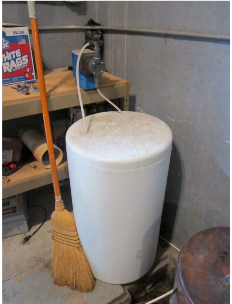
Photograph 10: Well 7 emergency chlorination components
