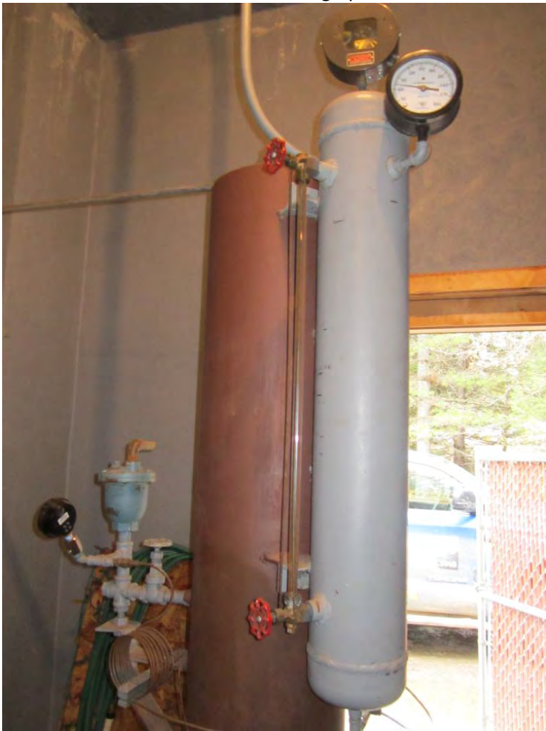
Photograph 7: Well 7 air/pressure release (torpedo casing)
