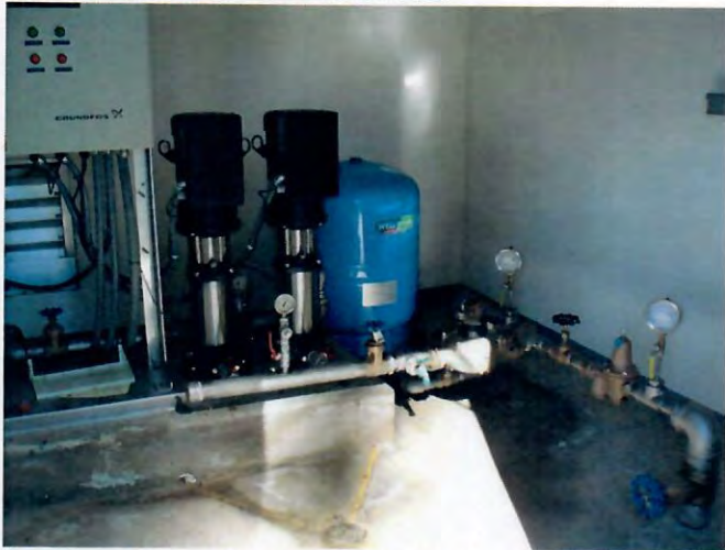
Photograph 14: Pend Orielle Pines booster pumps
