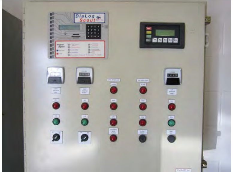
Photograph 68: Limekiln booster pump controls
