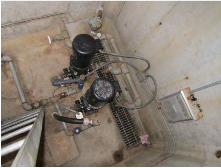
Photograph 53: Dromore booster pumps
