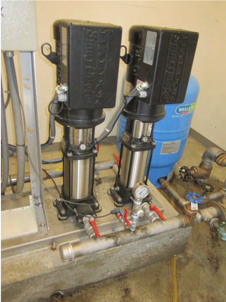
Photograph 59: Pend Oreille booster pumps
