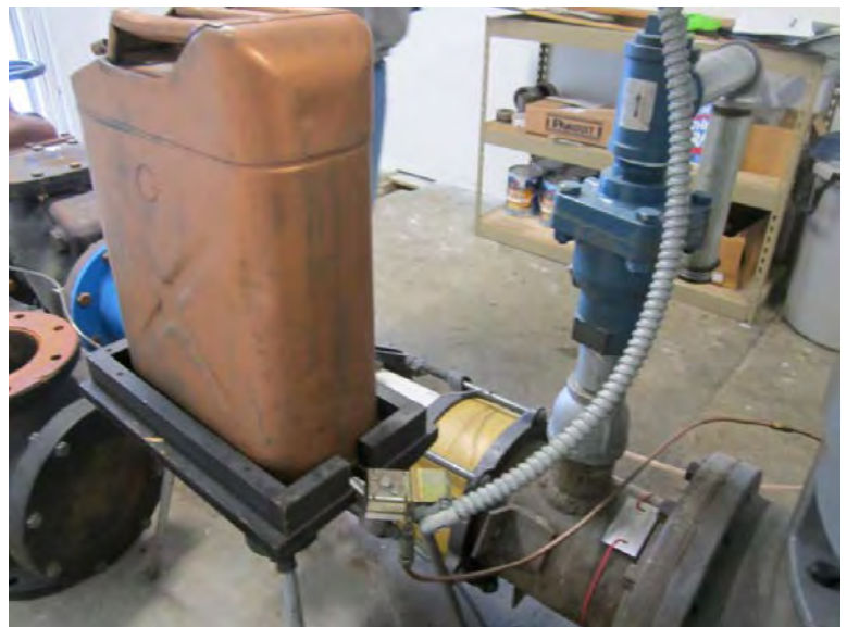
Photograph 18: Well 8 discharge appurtenances
