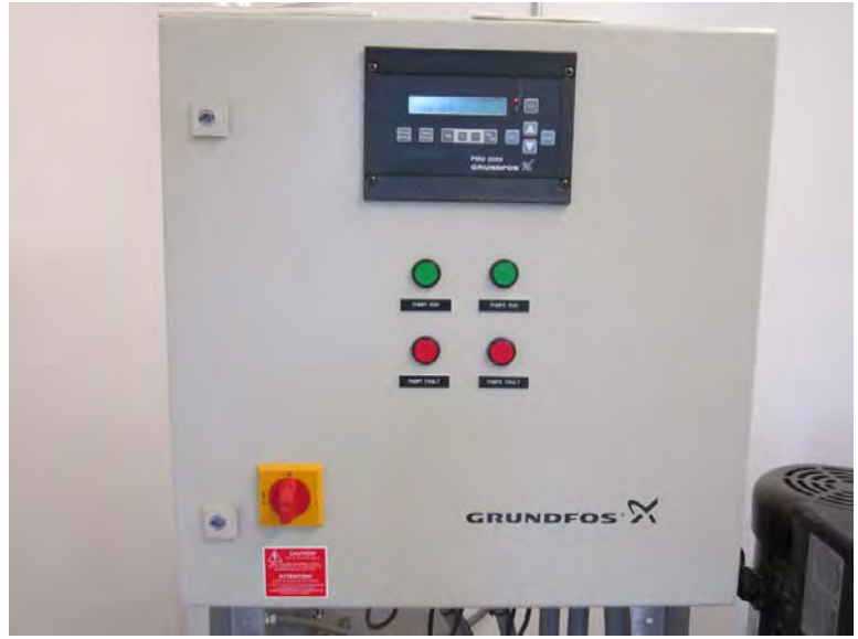
Photograph 58: Pend Oreille tank VFD controls
