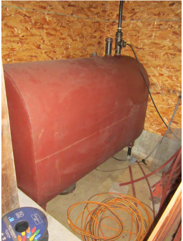
Photograph 12: Well 7 diesel fuel tank w/ secondary containment
