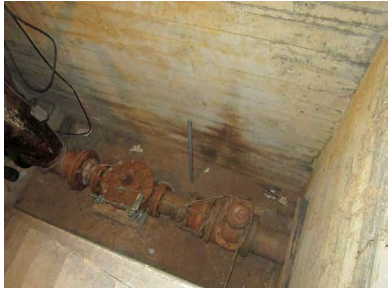
Photograph 46: Farragut tank PRV
