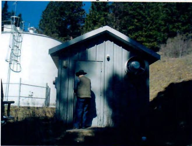
Photograph 13: Pend Orielle Pines Booster Station
