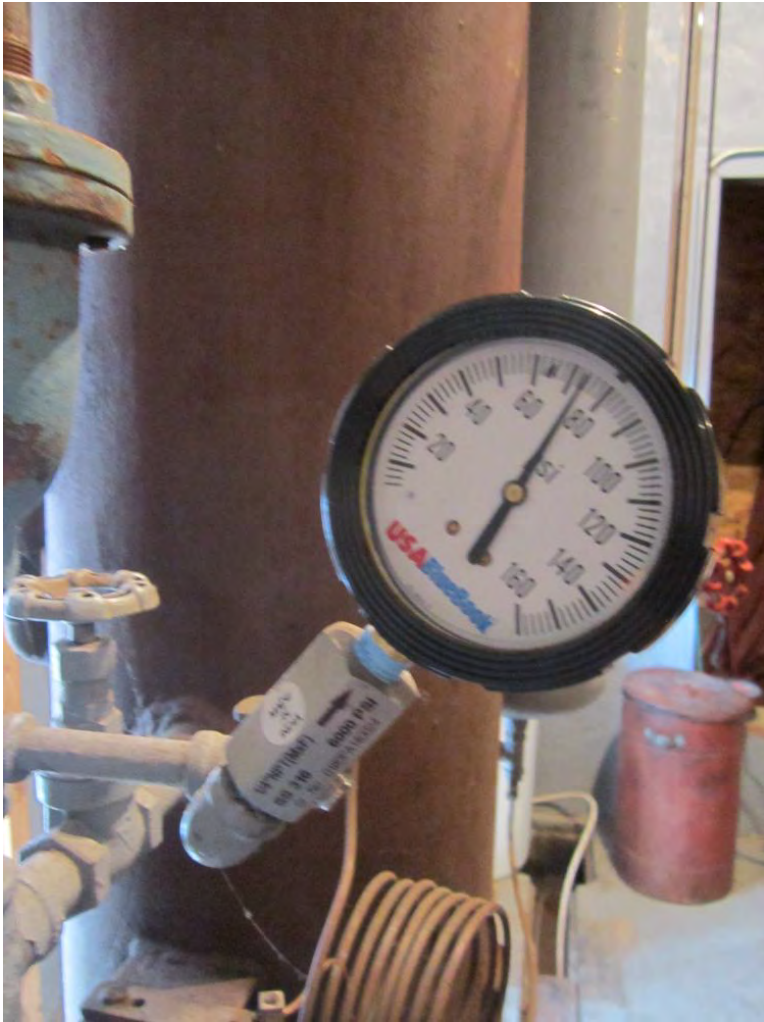
Photograph 9: Well 7 pressure gage
