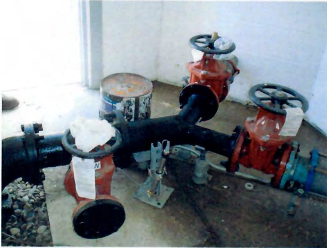
Photograph 19: Cape Horn Estates Reservoir valves
