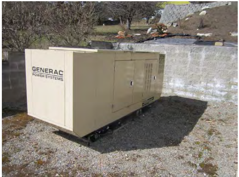
Photograph 64: Limekiln booster propane generator with auto-switchover
