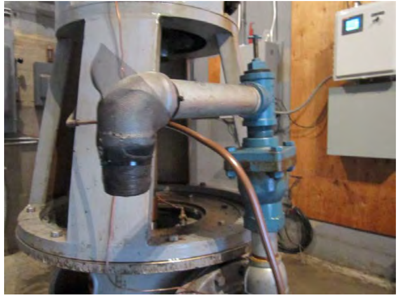
Photograph 4: Well 7 screened casing vent
