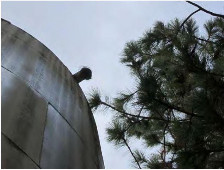
Photograph 45: Cape Horn tank screened vent/overflow 2
