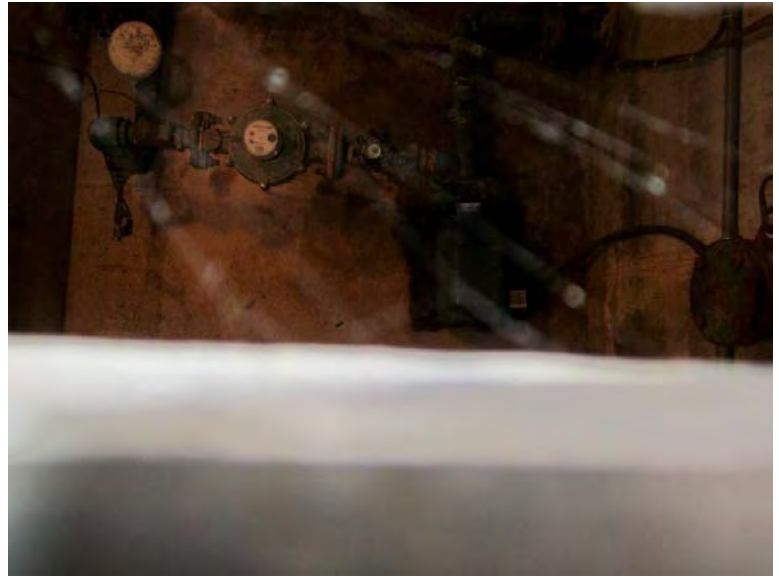
Photograph 38: Cape Horn booster station vault
