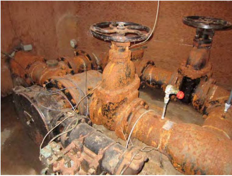
Photograph 31: Farragut Tank shared inflow/outflow isolation valves
