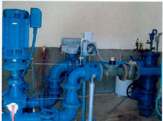
Photograph 10: Cape Horn Booster Pumps
