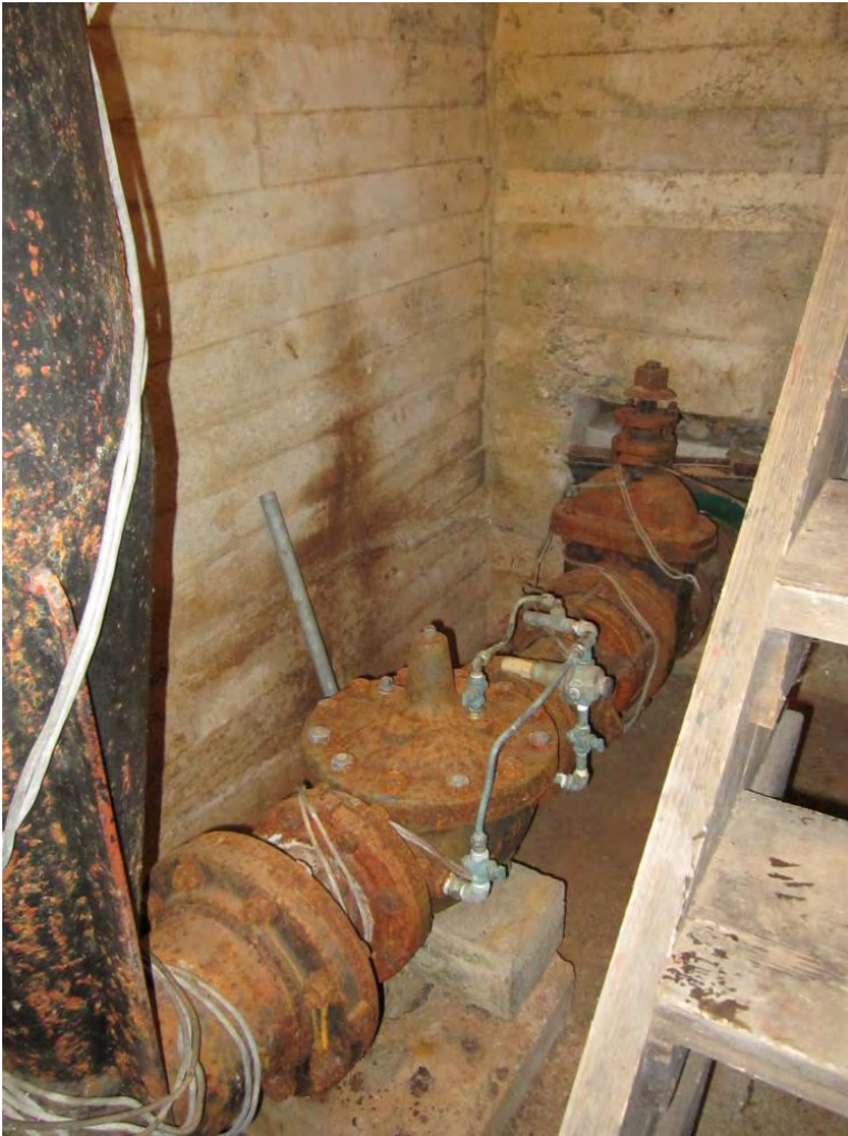
Photograph 49: Farragut tank PRV
