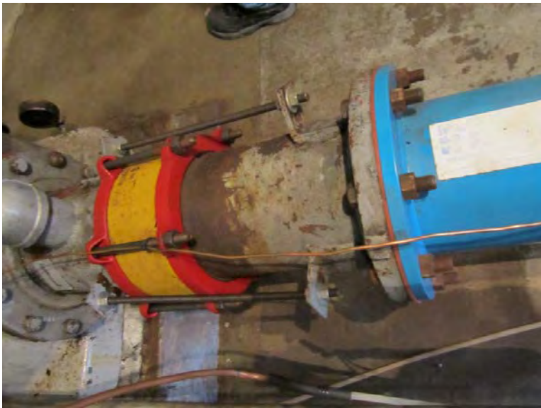
Photograph 5: Well 7 discharge appurtenances
