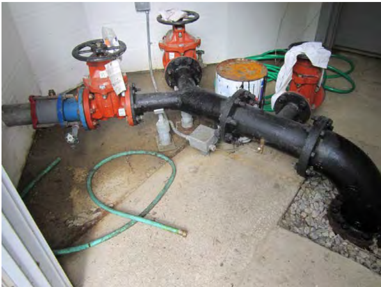
Photograph 43: Cape Horn tanks shared influent/effluent
