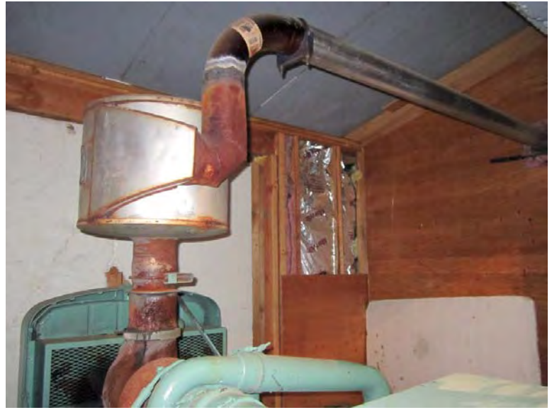
Photograph 2: Well 7 diesel manual switchover generator
