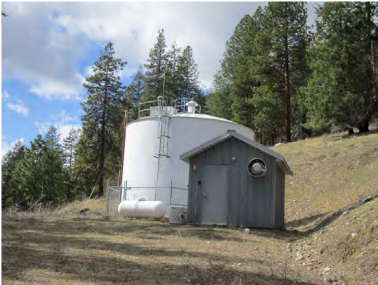
Photograph 55: Pend Oreille tank and booster station
