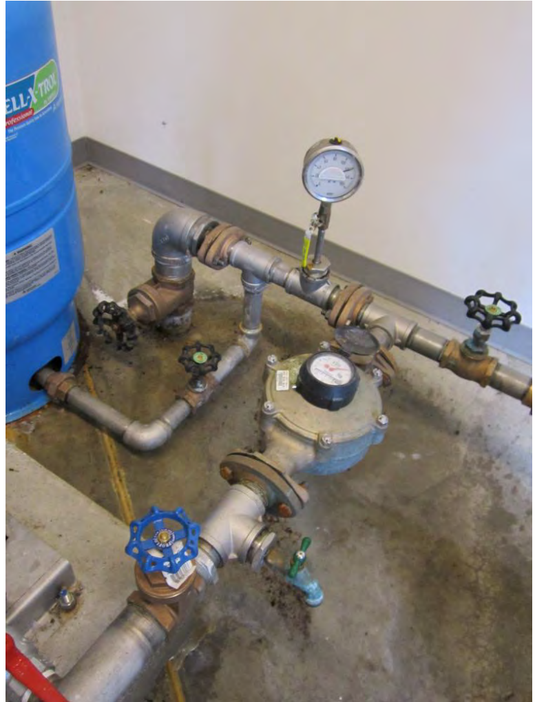
Photograph 60: Pend Oreille boosted discharge tee (PRV required on one tee)
