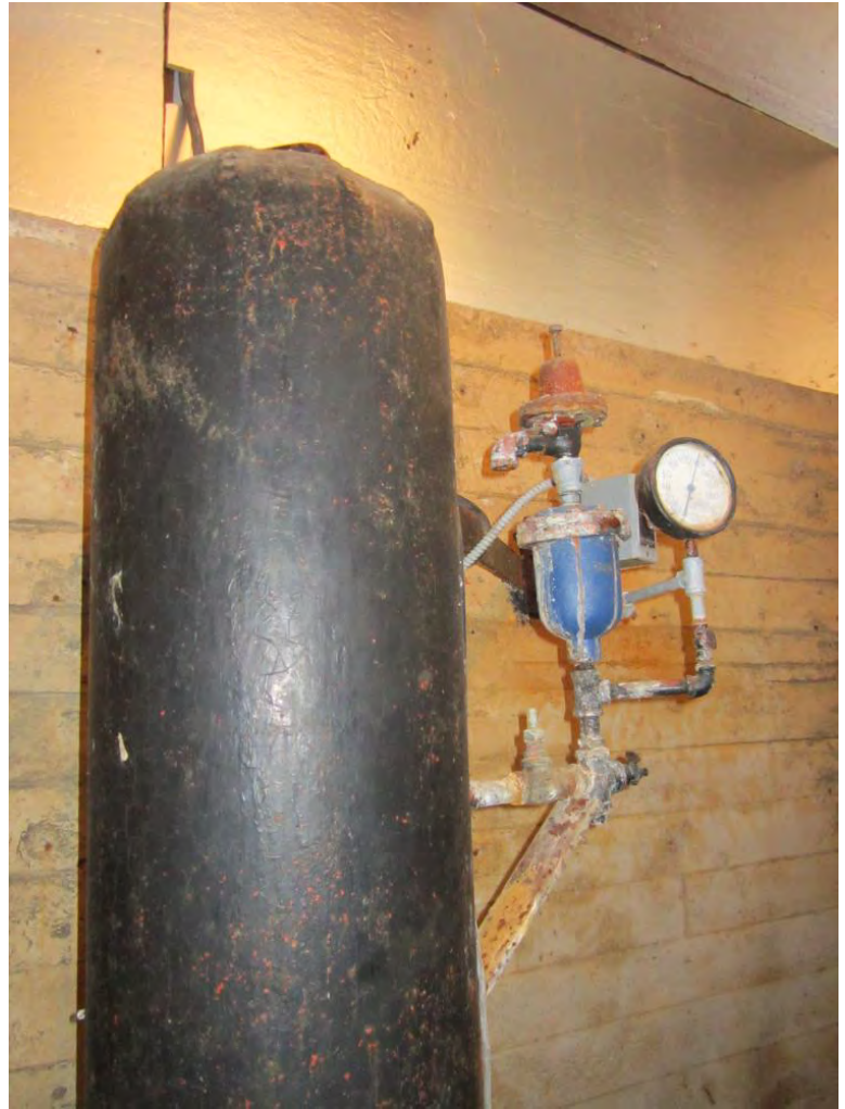
Photograph 50: Farragut tank PRV w torpedo casing pressure/air release
