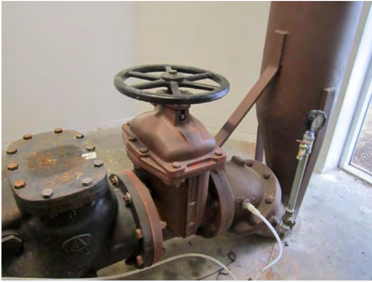
Photograph 21: Well 8 discharge appurtenances
