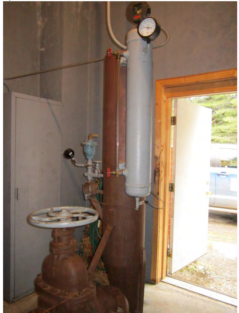
Photograph 8: Well 7 air/pressure relief (torpedo casing)
