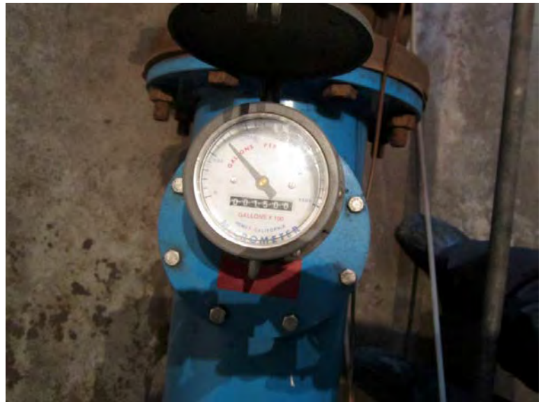
Photograph 6: Well 7 discharge appurtenances
