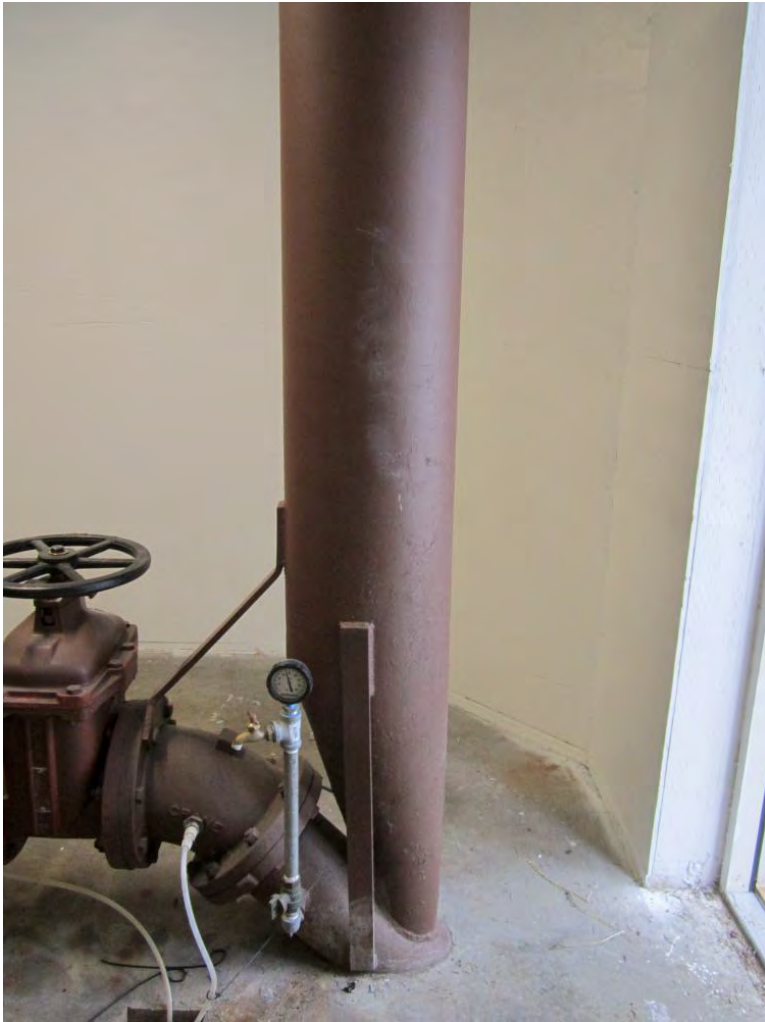
Photograph 19: Well 8 torpedo casing pressure/air release
