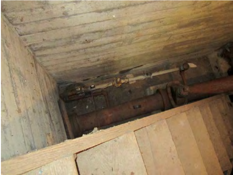
Photograph 47: Farragut tank PRV by-pass
