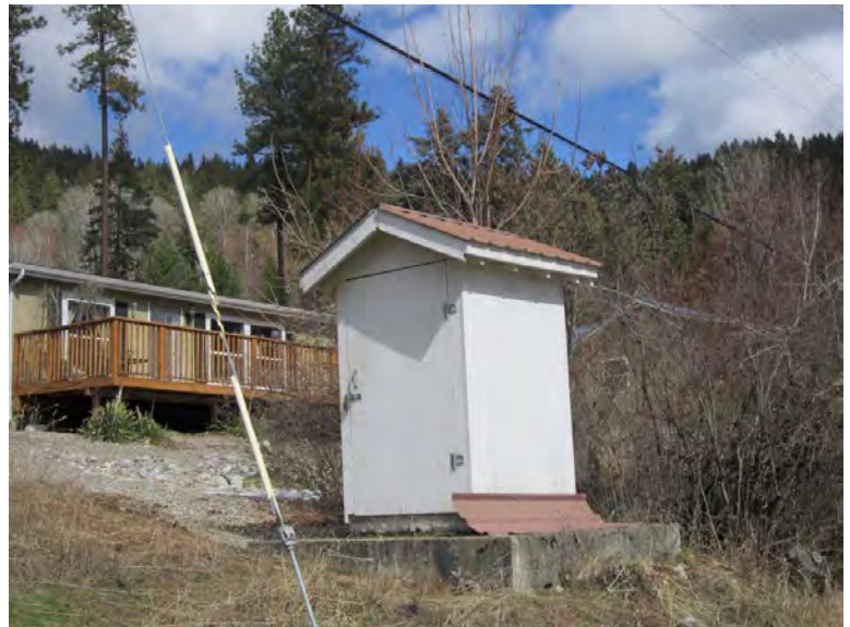
Photograph 52: Dromore booster station
