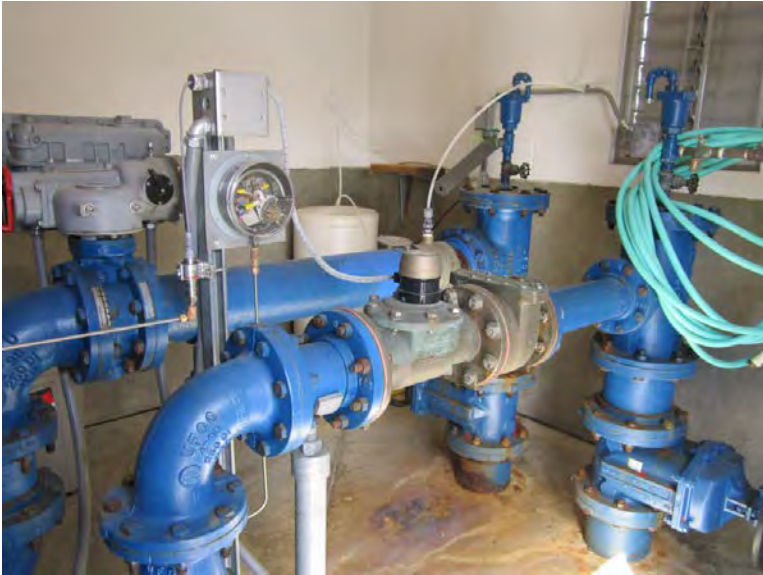
Photograph 67: Limekiln suction and boosted discharge lines
