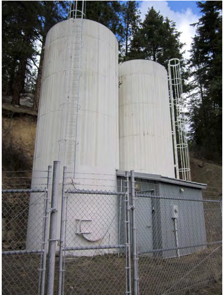
Photograph 42: Cape Horn tanks (30K each)
