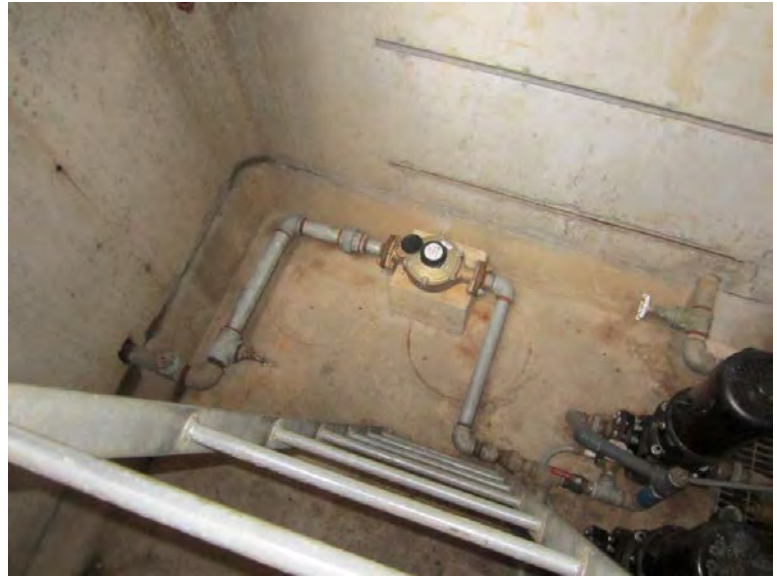
Photograph 54: Dromore booster pumps and flow meter
