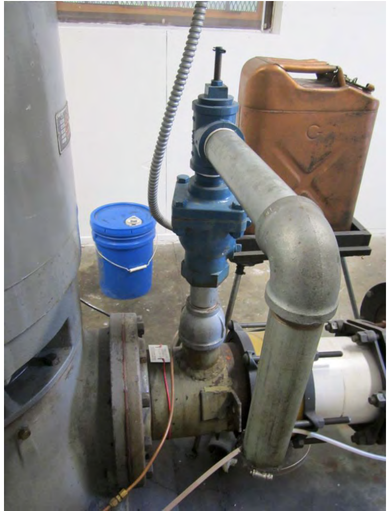
Photograph 16: Well 8 discharge appurtenances
