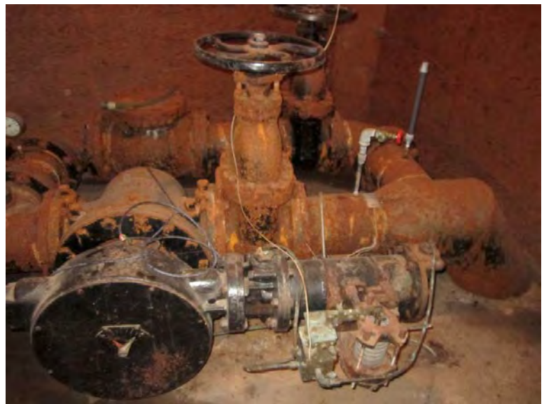
Photograph 30: Farragut Tank shared inflow/outflow isolation valves
