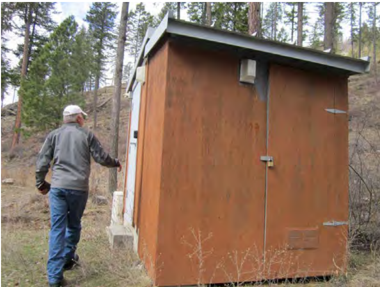
Photograph 35: Cape Horn Booster Station
