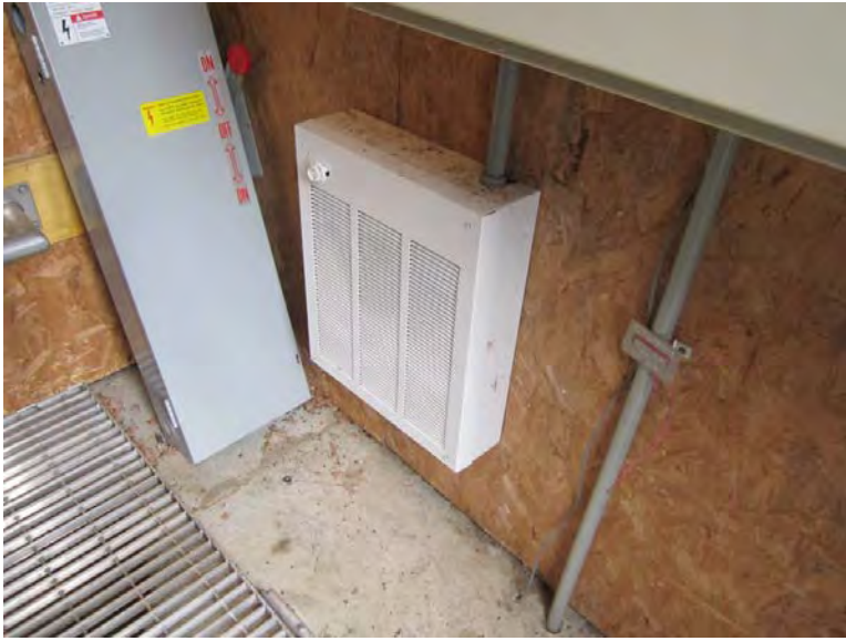
Photograph 41: Cape Horn booster station
