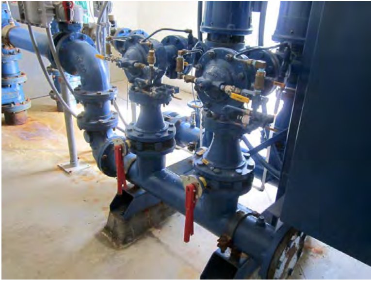
Photograph 69: Limekiln booster pump isolation valves
