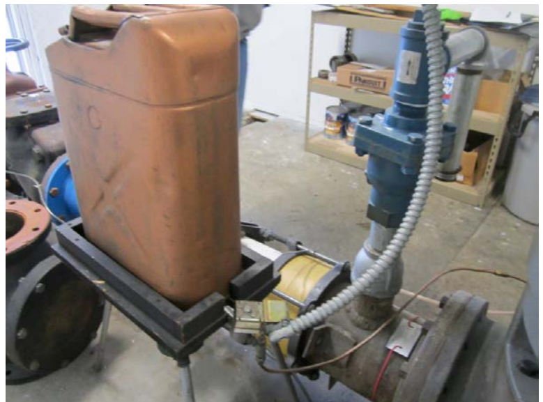
Photograph 18: Well 8 discharge appurtenances
