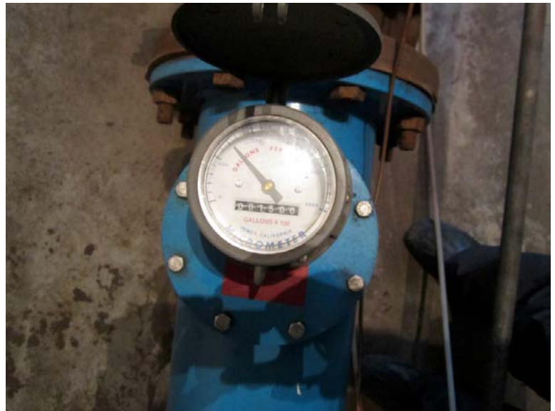
Photograph 6: Well 7 discharge appurtenances
