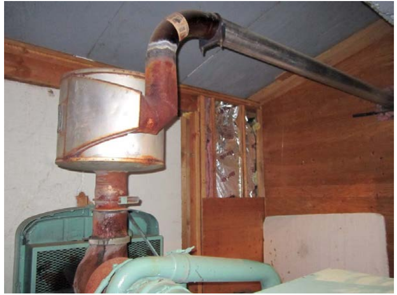
Photograph 2: Well 7 diesel manual switchover generator
