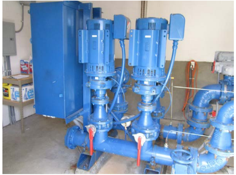
Photograph 66: Limekiln booster pumps
