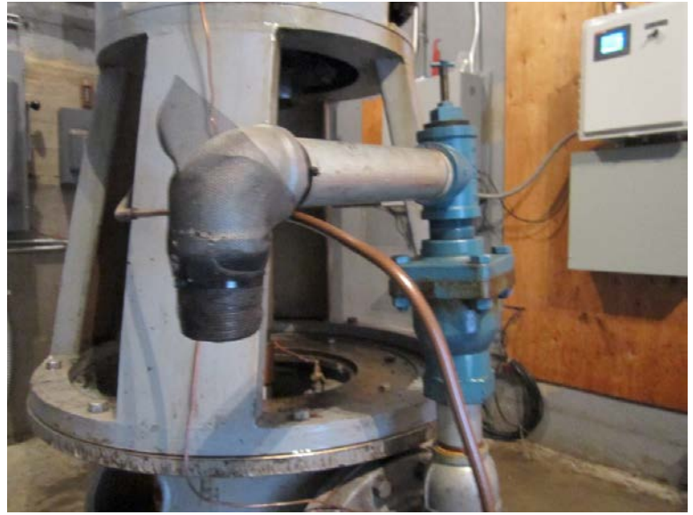
Photograph 4: Well 7 screened casing vent
