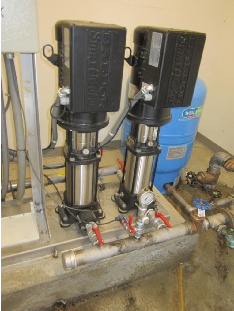
Photograph 59: Pend Oreille booster pumps
