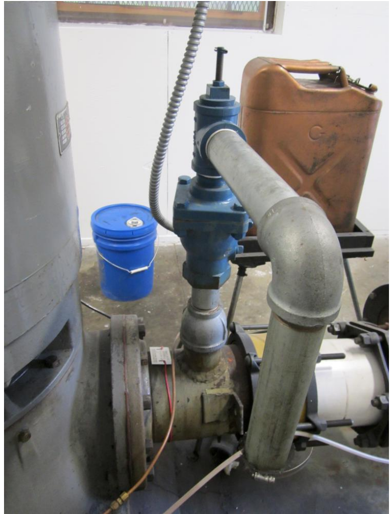
Photograph 16: Well 8 discharge appurtenances
