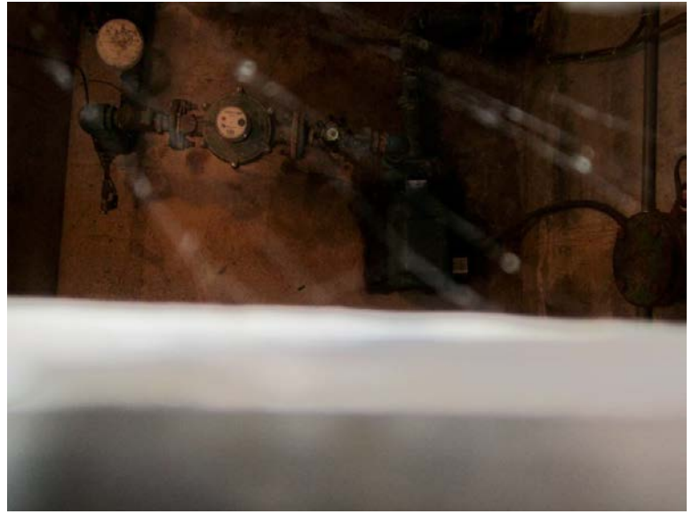
Photograph 38: Cape Horn booster station vault
