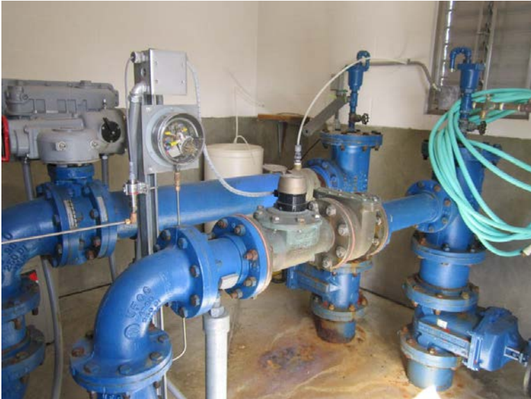
Photograph 67: Limekiln suction and boosted discharge lines
