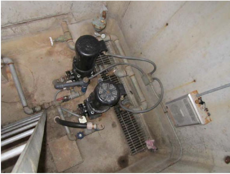
Photograph 53: Dromore booster pumps
