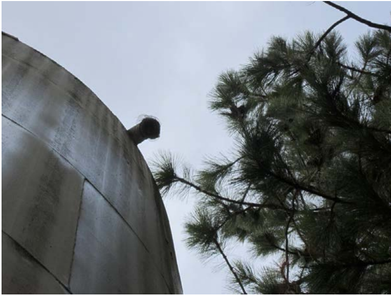
Photograph 45: Cape Horn tank screened vent/overflow 2
