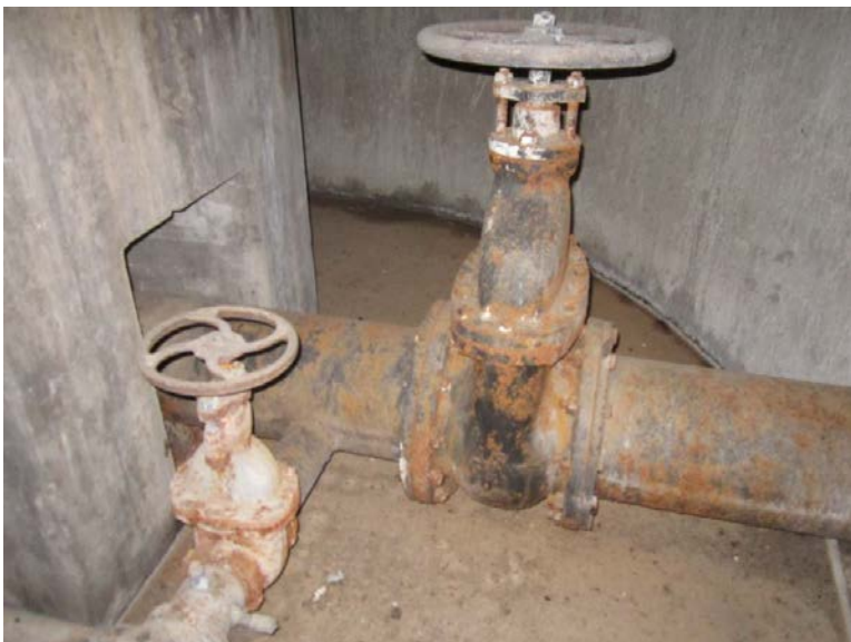
Photograph 29: Farragut Tank isolation valves
