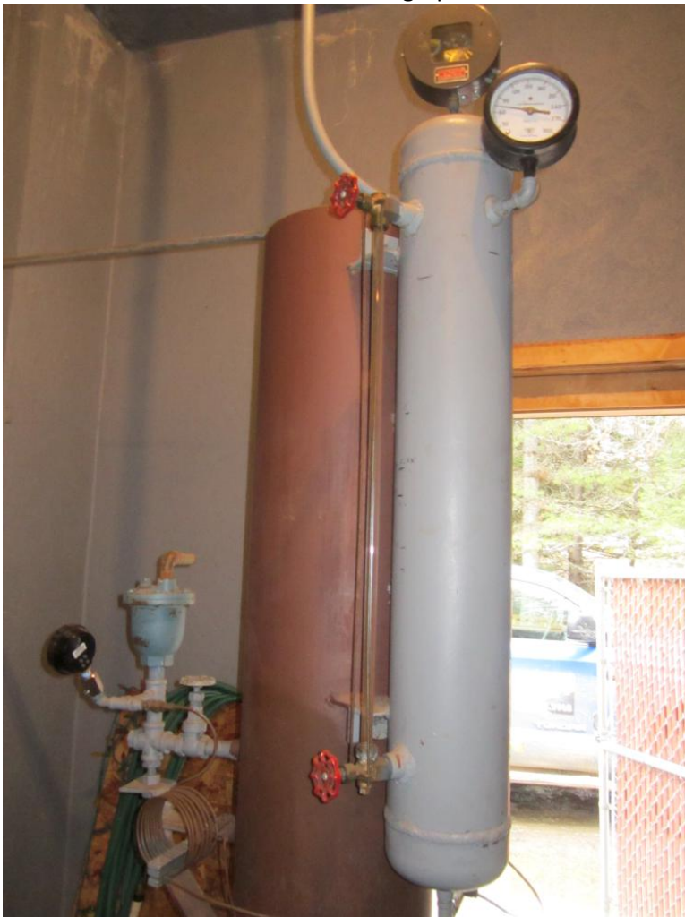
Photograph 7: Well 7 air/pressure release (torpedo casing)
