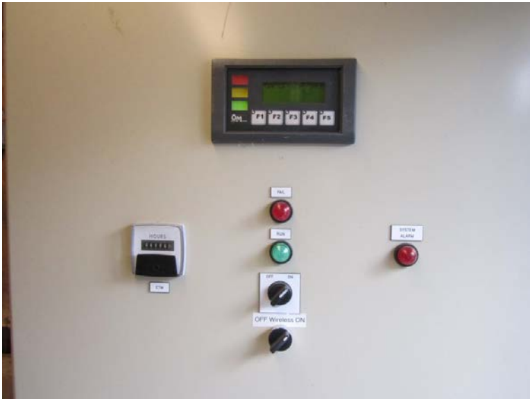
Photograph 39: Cape Horn booster station vault
