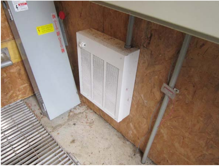
Photograph 41: Cape Horn booster station
