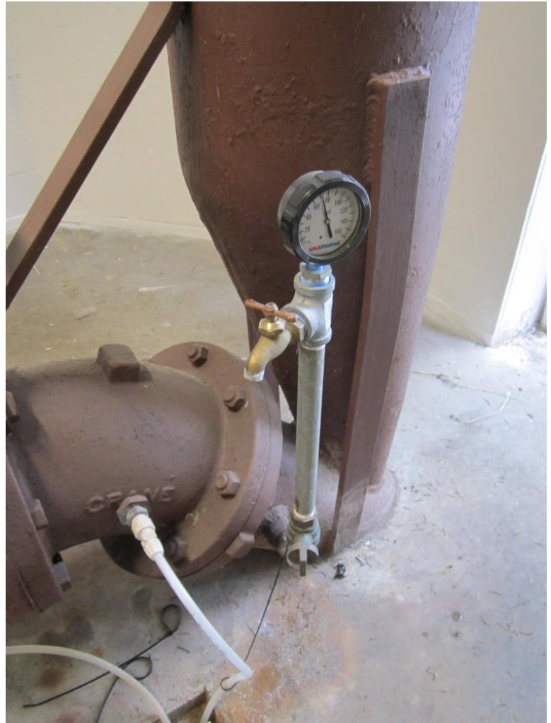
Photograph 20: Well 8 discharge appurtenances
