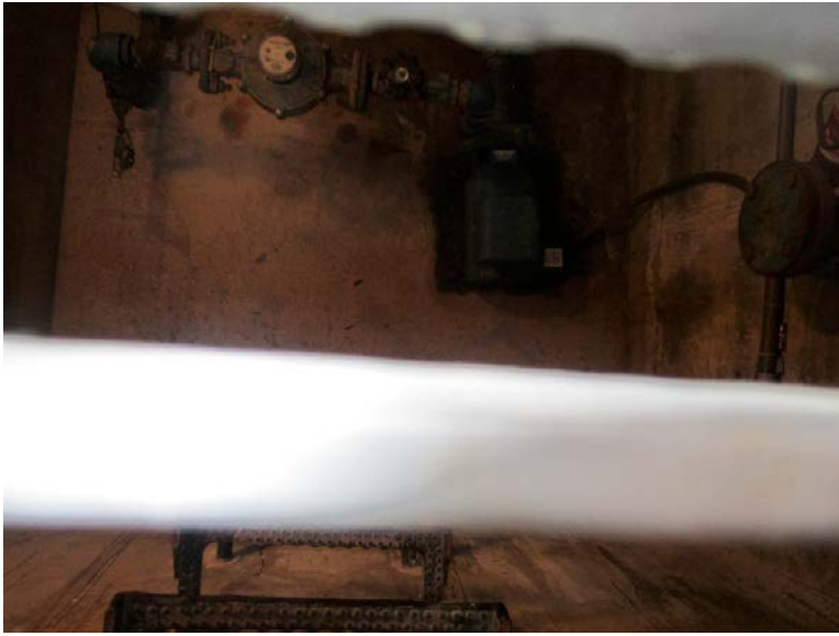
Photograph 37: Cape Horn booster station vault
