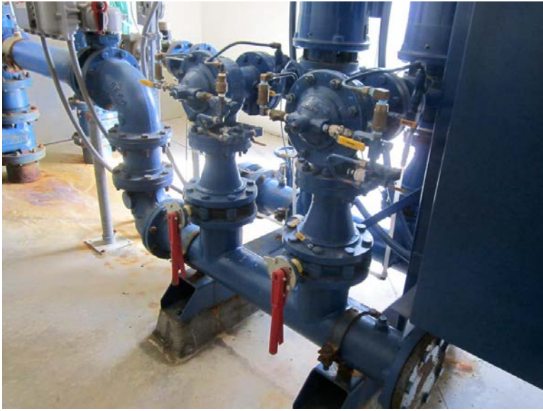
Photograph 69: Limekiln booster pump isolation valves
