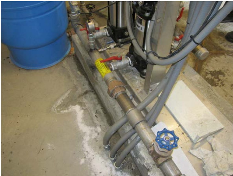
Photograph 63: Pend Oreille booster pump isolation valves
