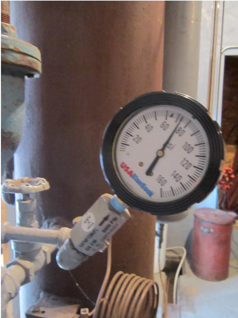
Photograph 9: Well 7 pressure gage
