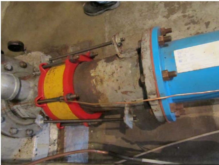
Photograph 5: Well 7 discharge appurtenances
