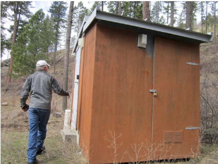
Photograph 35: Cape Horn Booster Station
