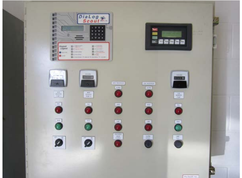
Photograph 68: Limekiln booster pump controls
