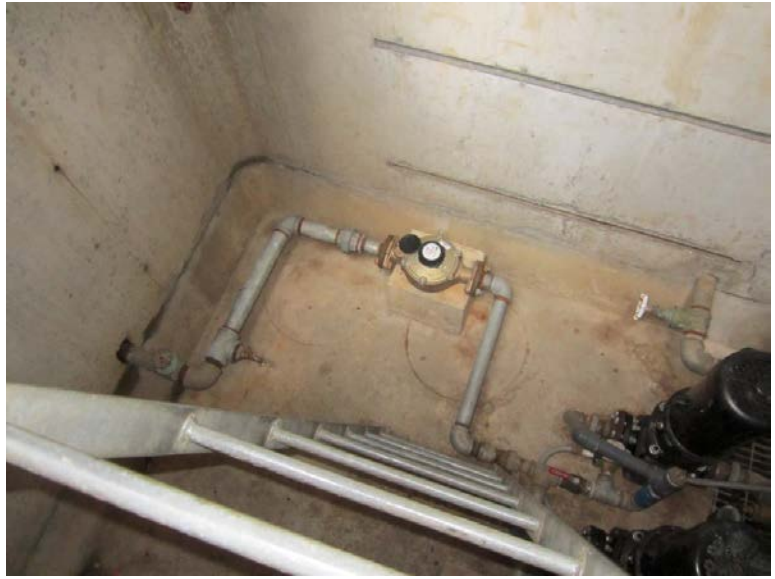
Photograph 54: Dromore booster pumps and flow meter
