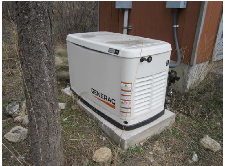
Photograph 36: Cape Horn booster station propane generator w auto-switchover
