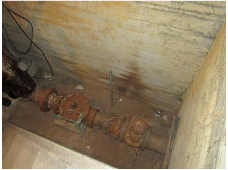
Photograph 46: Farragut tank PRV
