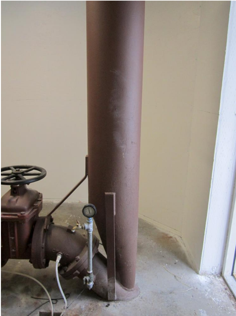
Photograph 19: Well 8 torpedo casing pressure/air release
