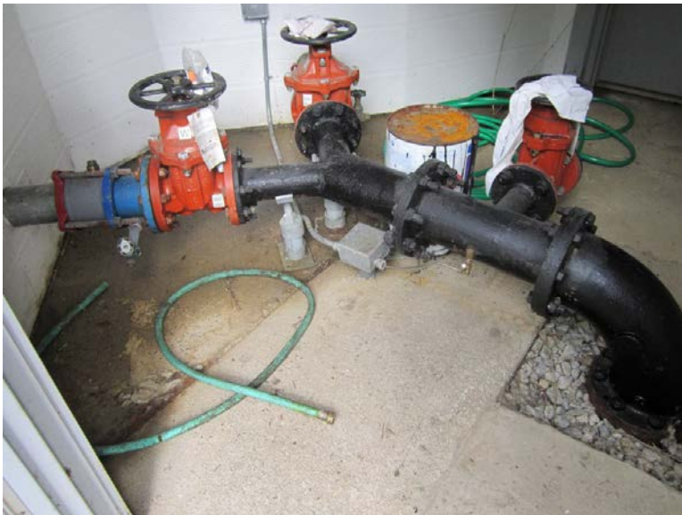
Photograph 43: Cape Horn tanks shared influent/effluent
