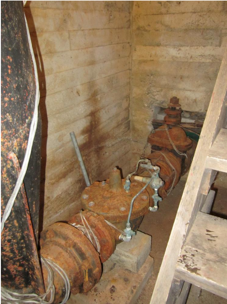
Photograph 49: Farragut tank PRV
