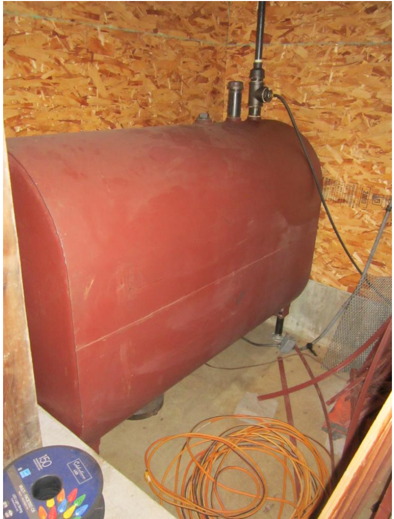
Photograph 12: Well 7 diesel fuel tank w/ secondary containment
