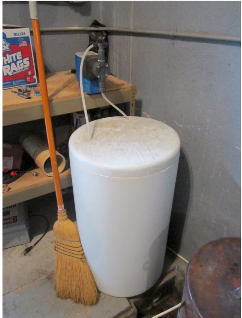
Photograph 10: Well 7 emergency chlorination components
