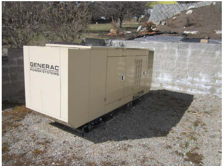
Photograph 64: Limekiln booster propane generator with auto-switchover
