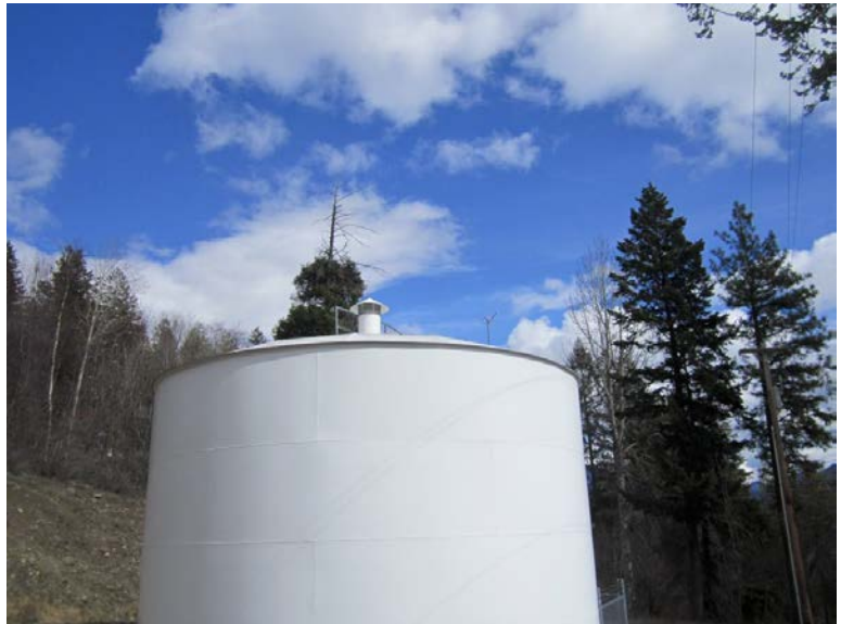
Photograph 56: Pend Oreille tank vent w screen
