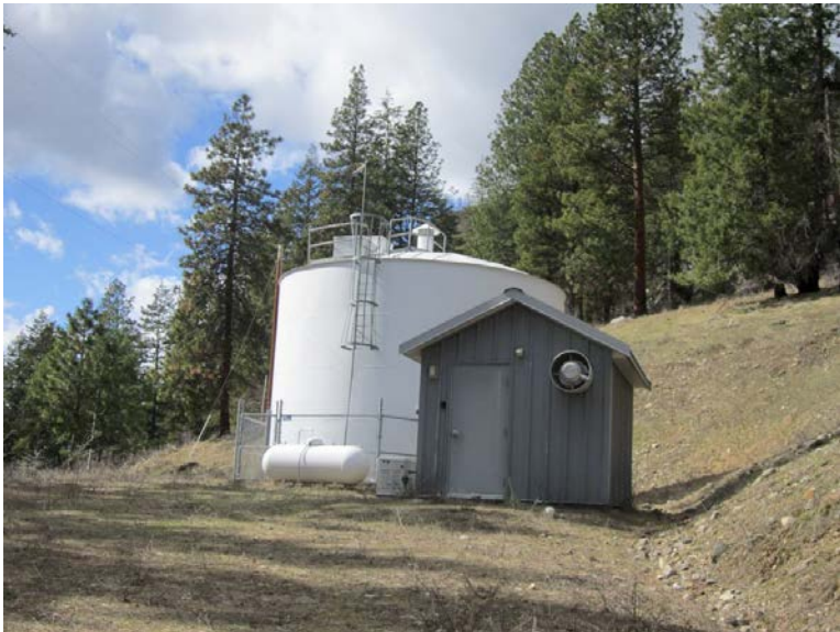
Photograph 55: Pend Oreille tank and booster station
