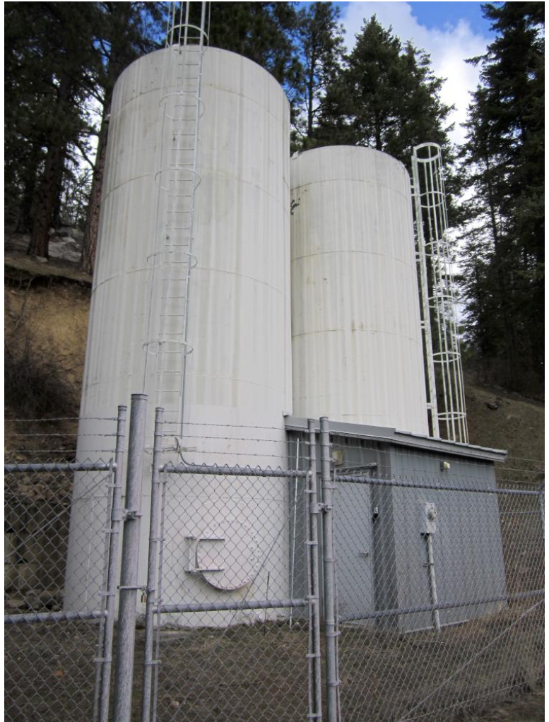
Photograph 42: Cape Horn tanks (30K each)
