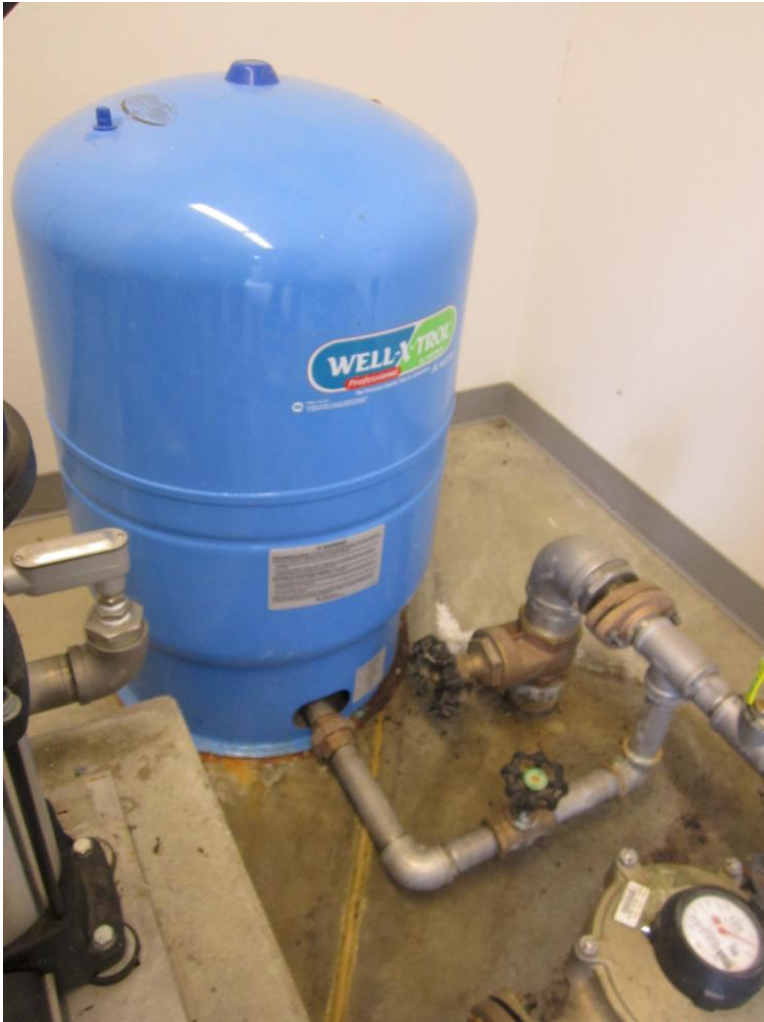
Photograph 61: Pend Oreille boosted discharge (hydro tank waterlogged)
