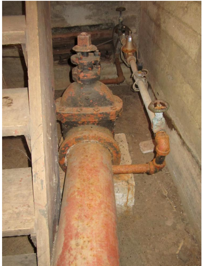
Photograph 48: Farragut tank PRV by-pass
