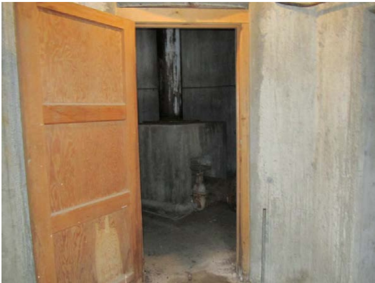
Photograph 25: Farragut Tank shared inflow/outflow
