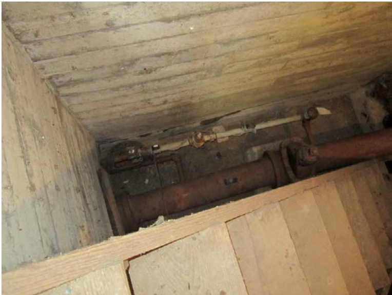
Photograph 47: Farragut tank PRV by-pass
