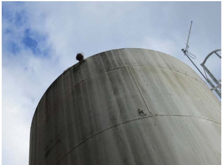
Photograph 44: Cape Horn tank screened vent/overflow 1
