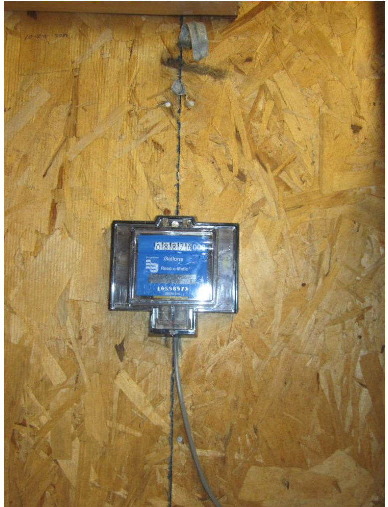
Photograph 40: Cape Horn booster station flow meter
