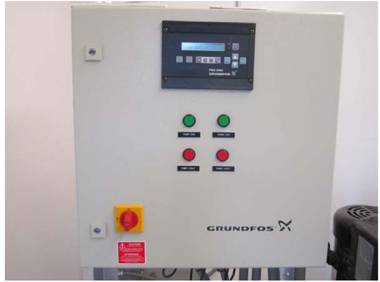
Photograph 58: Pend Oreille tank VFD controls
