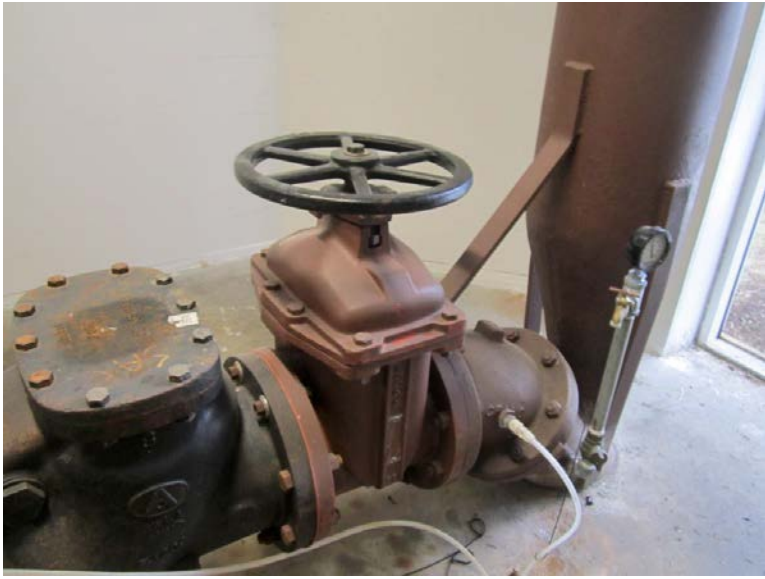
Photograph 21: Well 8 discharge appurtenances
