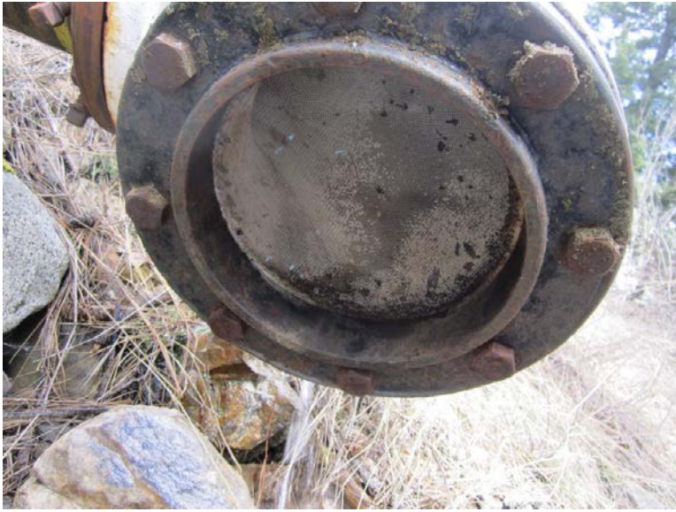
Photograph 57: Pend Oreille tank overflow
