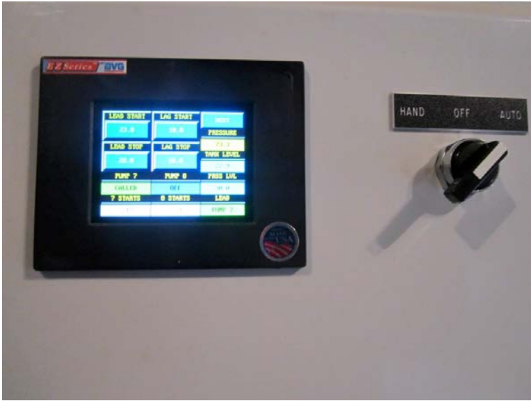
Photograph 11: Well 7 PLC tied to SCADA relay
